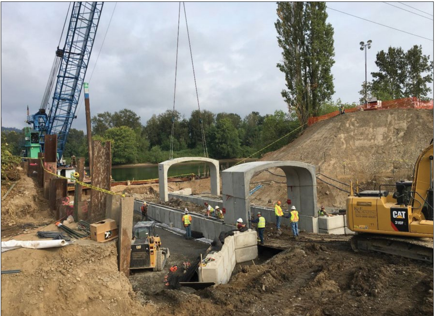
A crane lifts one of the culvert sections into place. The precast culvert pieces were formed off-site and brought in by barge to allow for faster assembly and to decrease the project's footprint.
