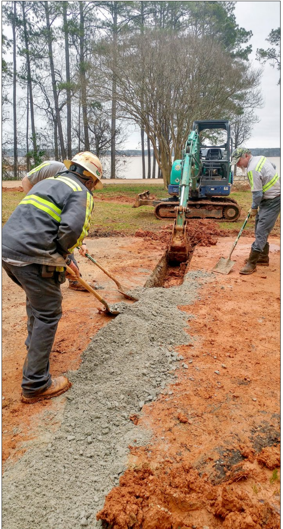
Contractors install a new water line at Whitetail Ridge Campground on the western shore of West Point Lake along the Alabama-Georgia state line. (Photo courtesy of West Point Project)
