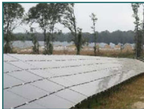
Fort Rucker 10 MW Large-Scale Renewable Energy Solar Project (April 2017)
