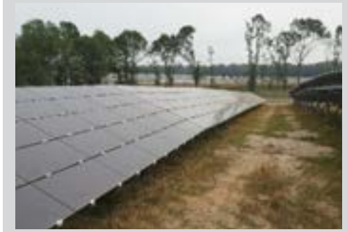
Fort Rucker, Ala. 10 MW Solar Renewable Energy Project Ribbon Cutting Event: April 20
