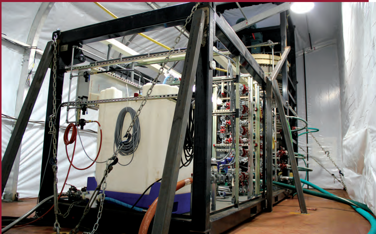
One of two FDHS units installed under engineering controls into the MV Cape Ray to destroy Syria's chemical weapons at sea.
