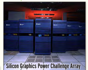
Silicon Graphics Power Challenge Array
