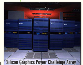
Silicon Graphics Power Challenge Array
