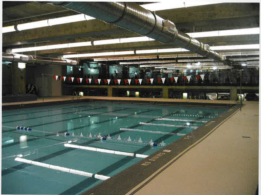
The new Pentagon Athletic Center pool is twice the size of the former pool and features a new technology ozone chlorinating system.
