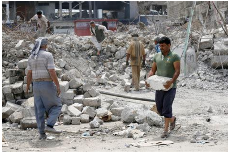
Figure 2: Mosul Civilians Helping to Clear Debris
