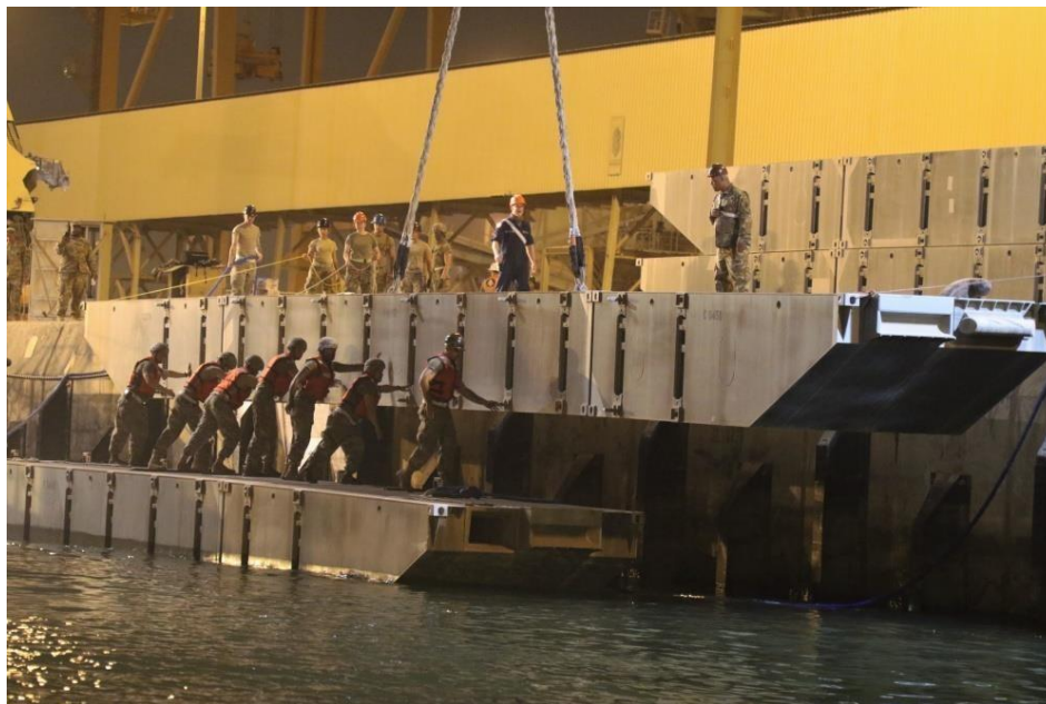
SHUAIBA PORT, Kuwait – Members of the 331st Transportation Company work with the 38th Sustainment Brigade to use the barge derrick crane to hoist strings into the port so that they can build the roll-on/roll-off discharge facilities for the LOTS mission during NH18. (U.S. Army Photo by Staff Sgt. Charlotte Reavis).
