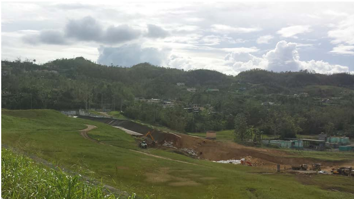
Figure 1- 4 Soldiers and the U.S. Army Corps of Engineers repair damage to the Guajataca Dam.
