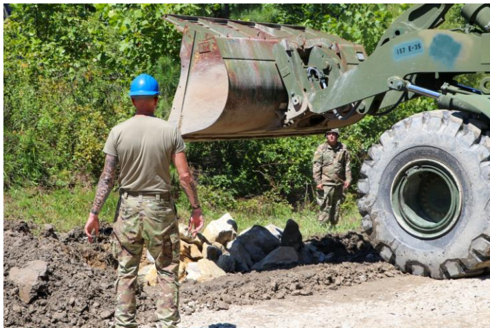
Virginia National Guard Soldiers assigned to the Blackstone-based 157th Engineer Platoon (Quarry), 276th Engineer Battalion, 329th Regional Support Group conduct quarry operations during their annual training Aug. 13, 2022, at Fort Pickett, Virginia. The 157th Engineer Platoon crushed rock which will be used to create protective berms and improve road surfaces on Fort Pickett ranges. Additional rock is stockpiled for use by the installation throughout the year.
