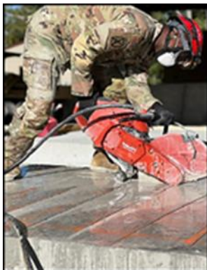
46th EN BN (20th EN BDE) cuts various structures to include concrete and masonry units ISO DCRF
