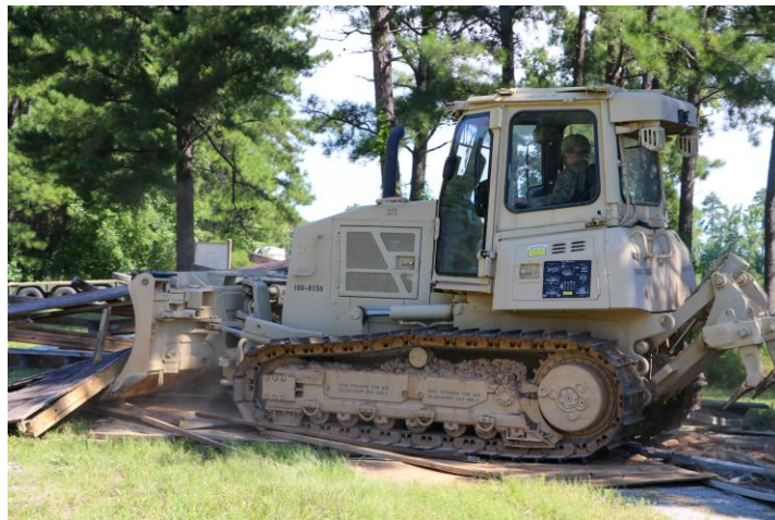
Virginia National Guard Soldiers assigned to the Powhatan-based 180th Engineer Support Company, 276th Engineer Battalion, 329th Regional Support Group conduct horizontal structure demolition during annual training Aug. 14, 2022, at Fort Pickett, Virginia. Engineers demolished wooden structures that have been used by the post since the early 2000s, making room for new buildings for future use.
